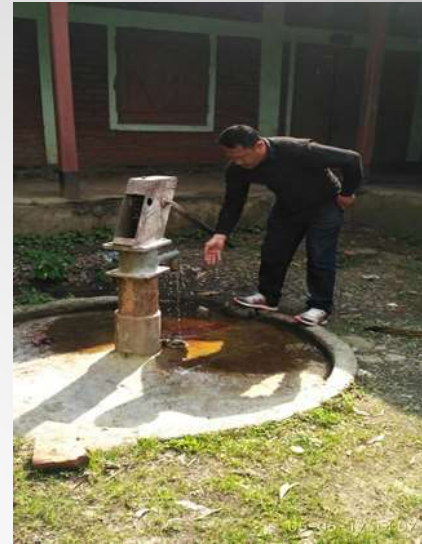
Iron contaminated hand pump in school
